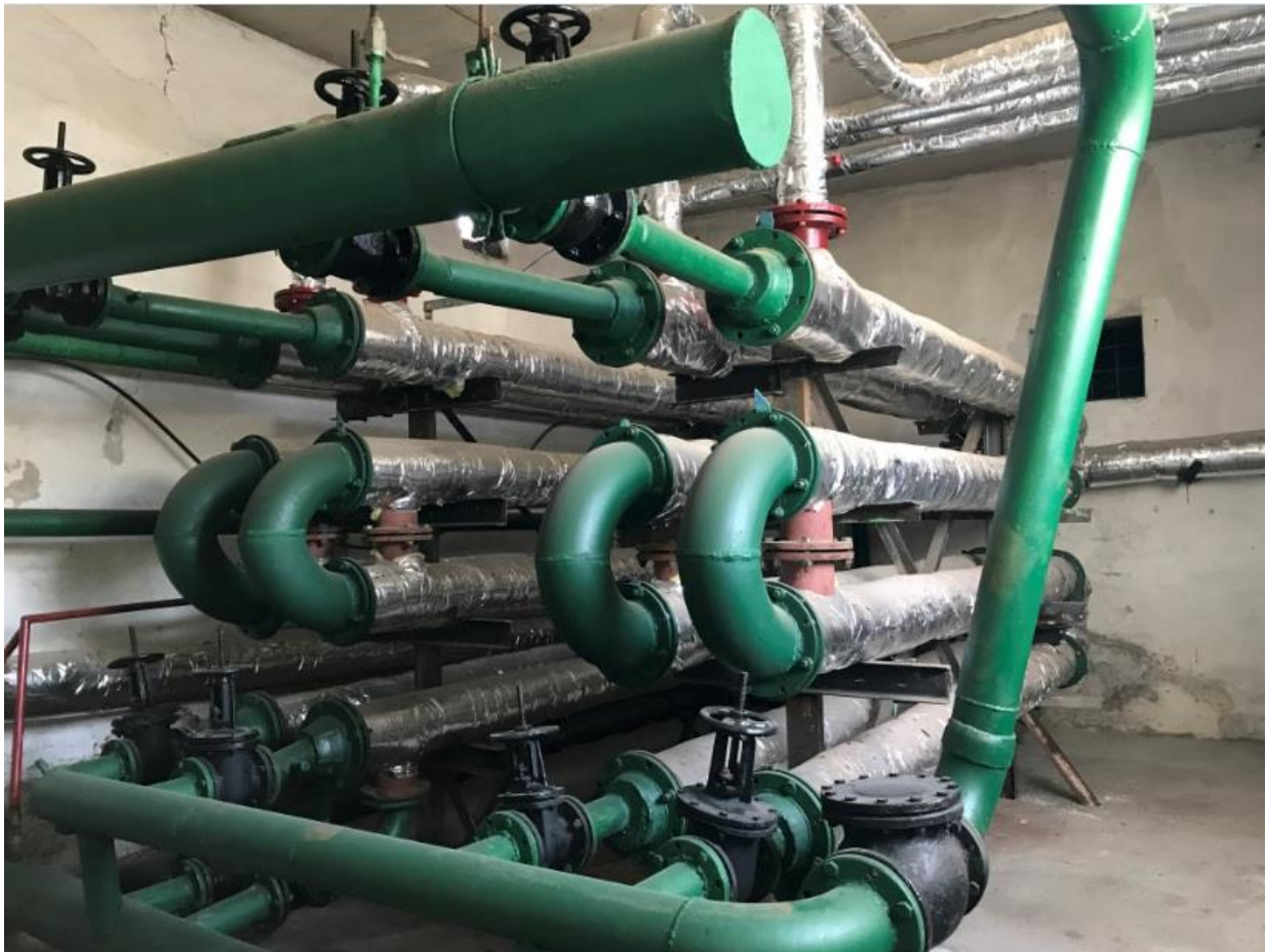
S-shaped pipes for heating and preventing water cooling
