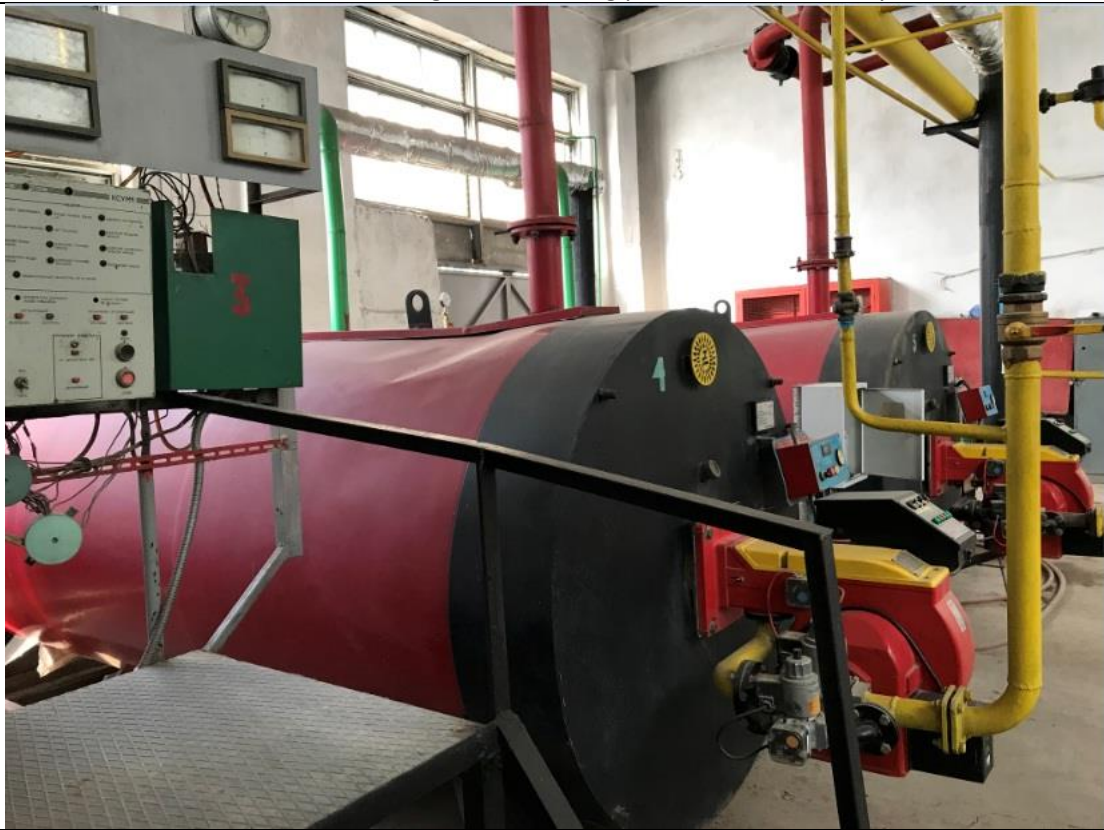
Swimming pool boilers
