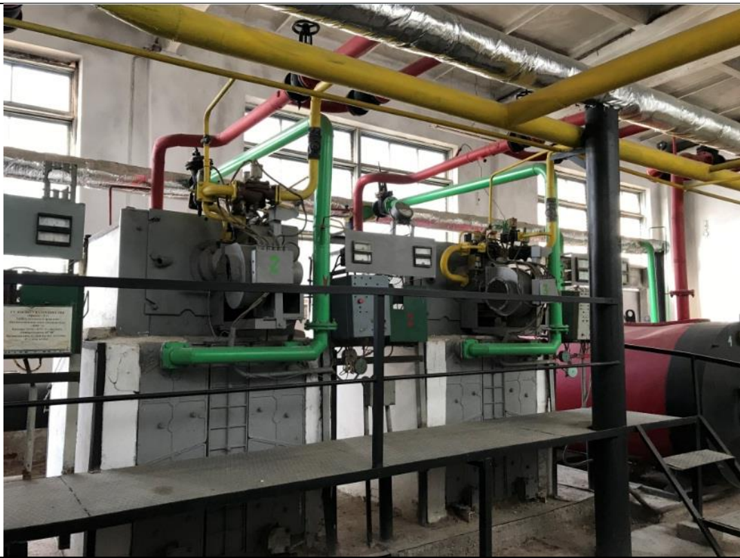
Installation serving the swimming pools of the university
