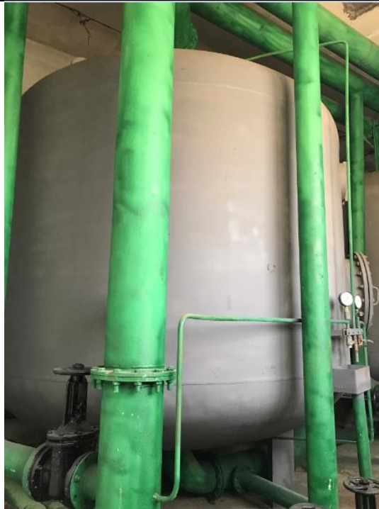
Large filters for water purification
