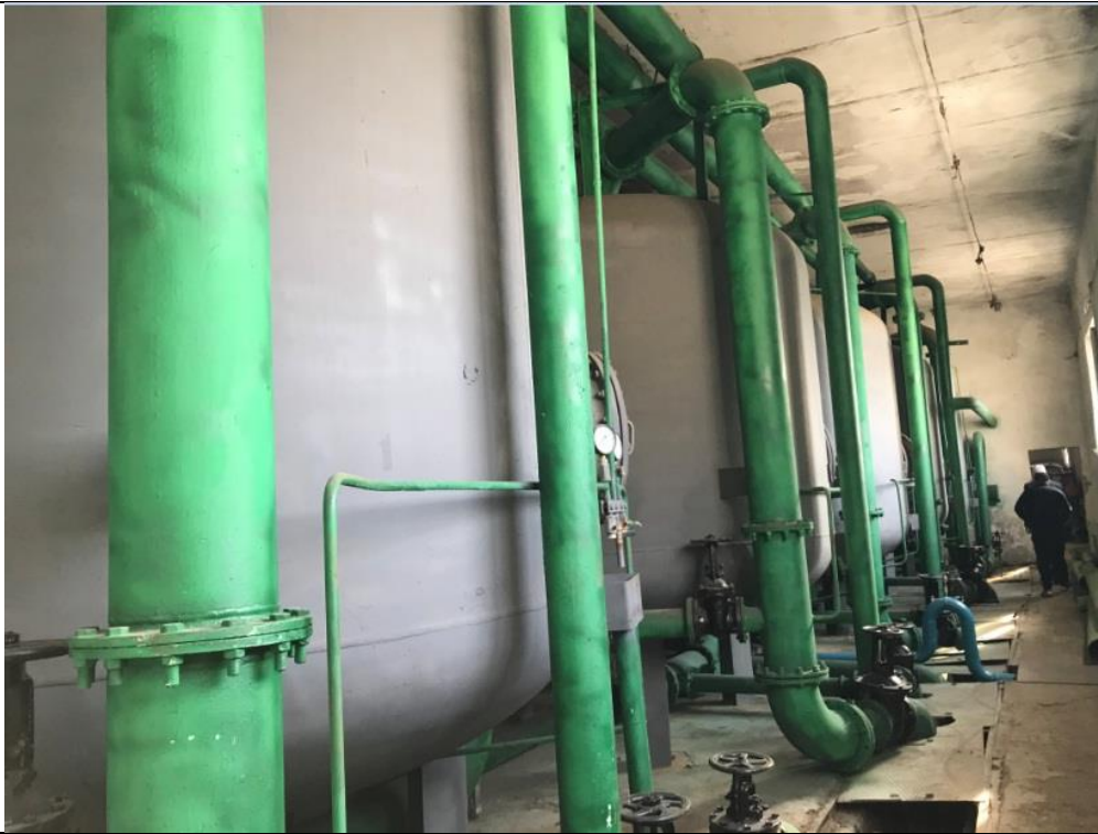
Water treatment plant with 4 filters
