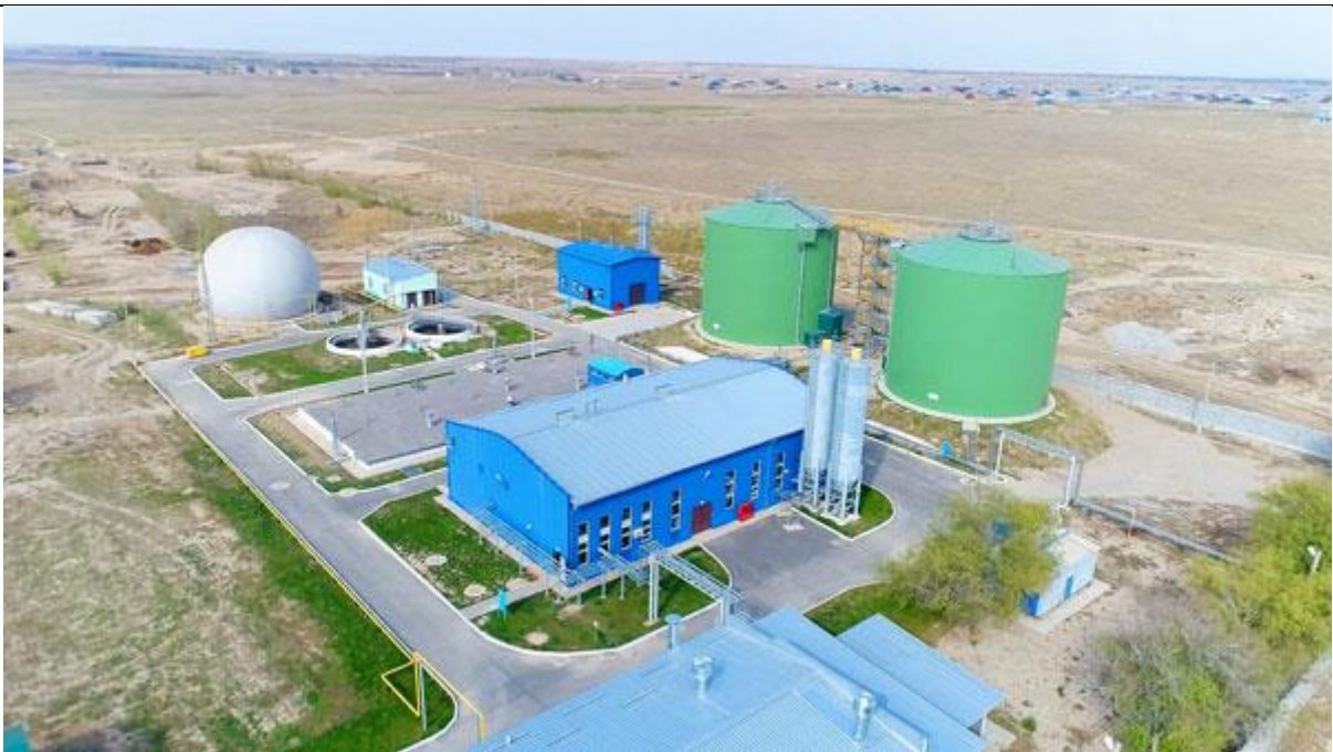
The final stage of water purification
