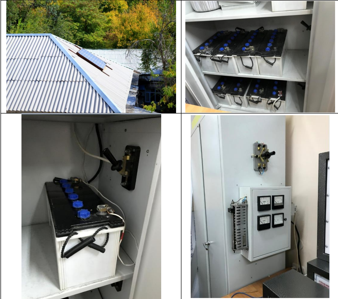
Campus 1. Solar battery (photo 1), rechargeable batteries (photo 2,3), transformer (photo 4).
