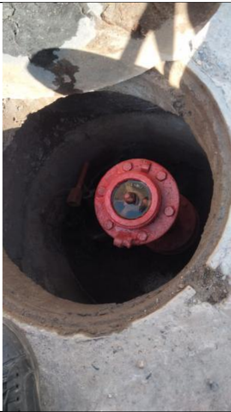
Underground fire hydrants
