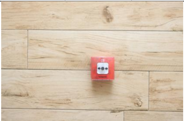
Fire alarm button
