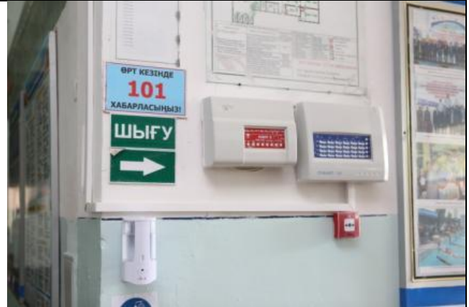
Alarm control panel in building 1
