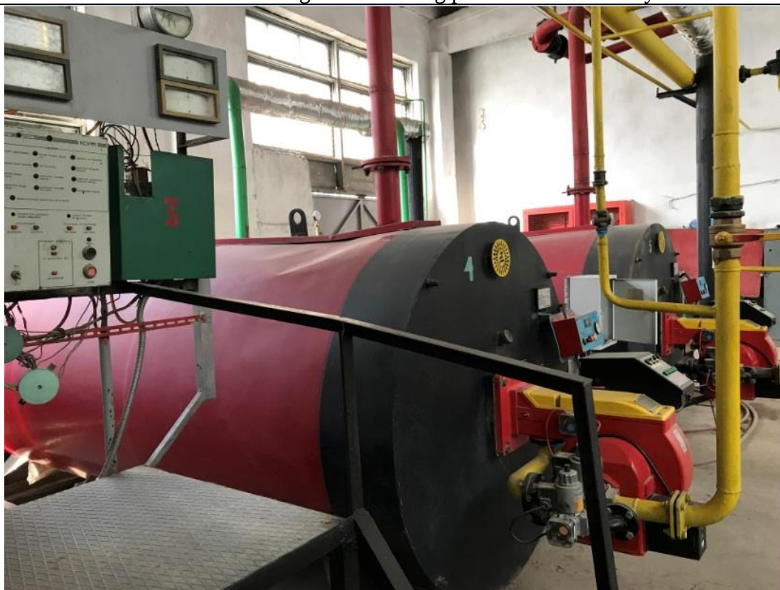
Swimming pool boilers
