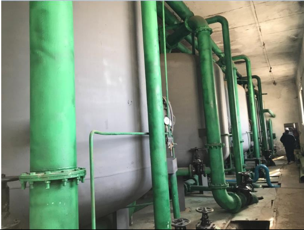
Water treatment plant with 4 filters
