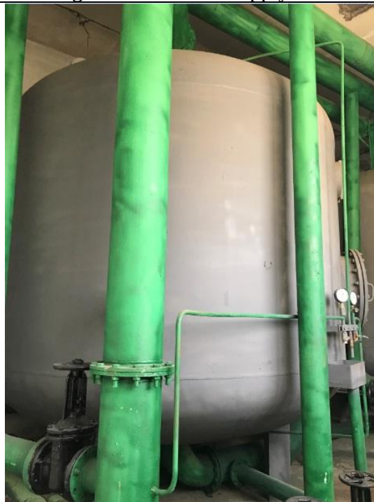
Large filters for water purification
